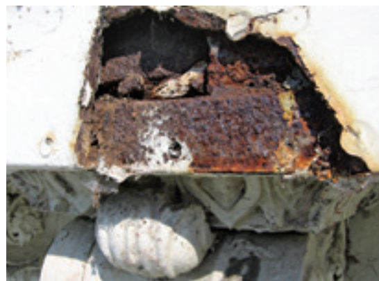
RUST TO DUST Significant portions of the cast iron dome have corroded and will need to be recast and replaced.
