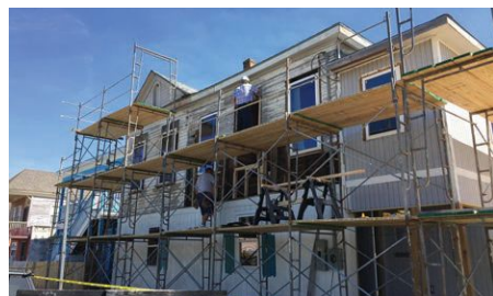
MobleySafway Solutions LLC recently donated $10,000 worth of scaffolding and labor to help Galveston Urban Ministries renovate its new office building.
